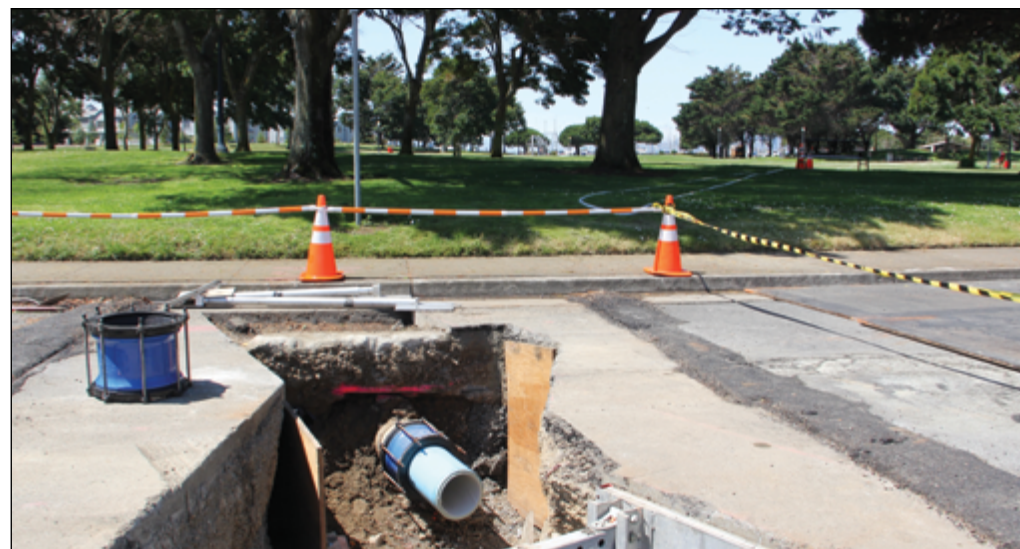
Marina Park in Richmond, where installation of Aqua-Pipe avoided the disruption to park services of extensive trenching. Photo: EBMUD
