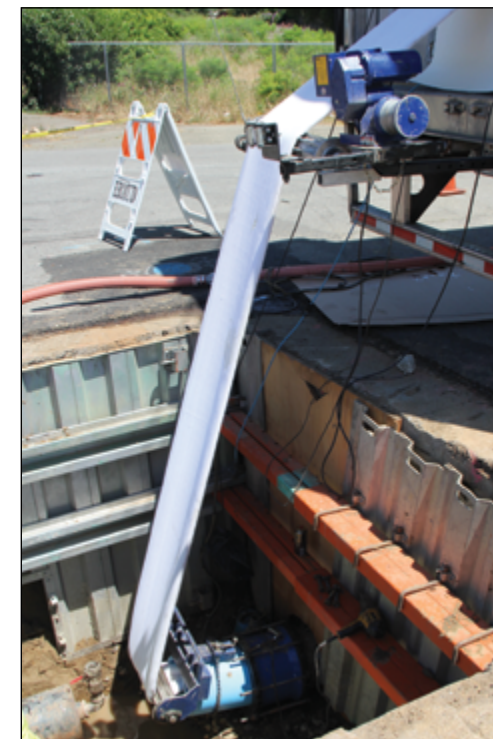
EBMUD feeds Aqua-Pipe sleeve liner from trailer into pipe, then injects resin while a winch pulls from the other end. The sleeve installed at Glenn Avenue in San Pablo was pulled 525 feet through a 12-inch asbestos cement pipe. Photos: EBMUD
