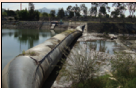
Rubber dam on Alameda creek. Photo: ACWD
