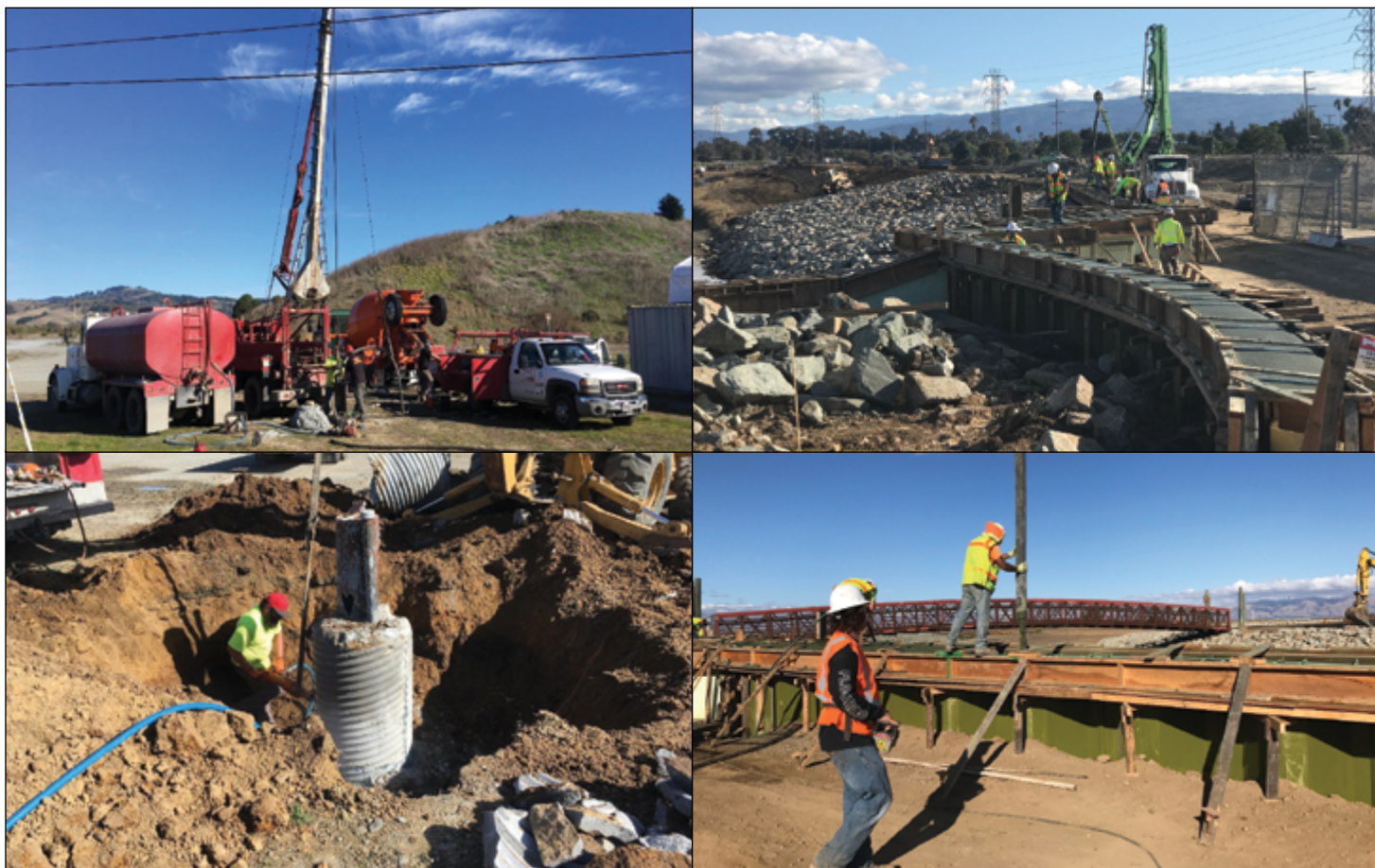
The state’s commitment to funding integrated regional water management is revealed in projects like this under construction in San Mateo County and along San Francisquito Creek in 2018. The SF Estuary Partnership is a key partner, as grant manager and regional collaborator, in achieving the multi-partner, multi-benefit “alignment” supported by DWR’s IRWM and the State Water Plan Update.
