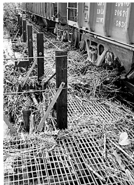
High flows deposit debris on a trestle over the Gualupe River. Photo courtesy Larry Johann.
