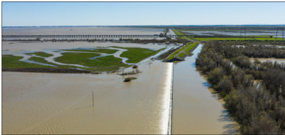
Fremont Weir, letting Sacramento River Water into the Yolo Bypass. Photo: Jak Wonderly
