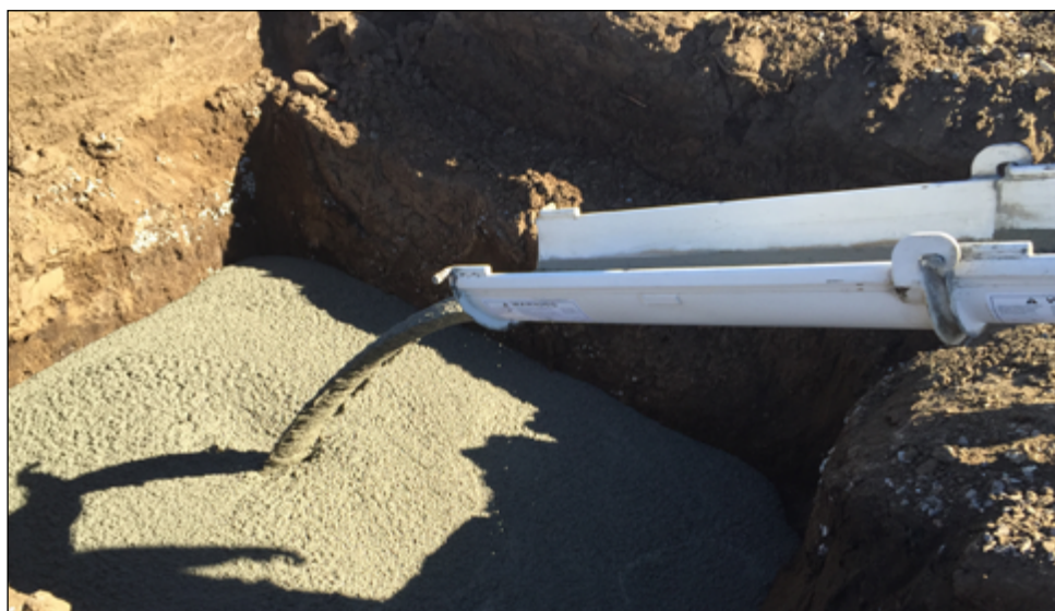
Backfilling the new sewer trench with a lean concrete slurry, which is stronger and less expensive than backfilling and compacting with soil. Photo: Sonoma Water
