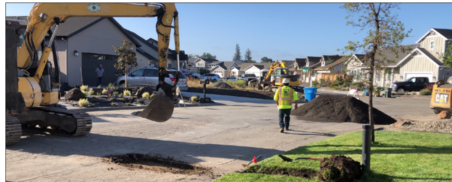
Connecting a sewer lateral. In some parts of the Larkfield project, contractors used a technique called trenchless installation to save cost. The technique involves drilling a small tunnel and pulling a long high-density polyethylene hose/pipe behind it. The driller aims the tunnel to a pit several hundred feet away where they connect to a conventional sewer pipe. Photo: Sonoma Water
