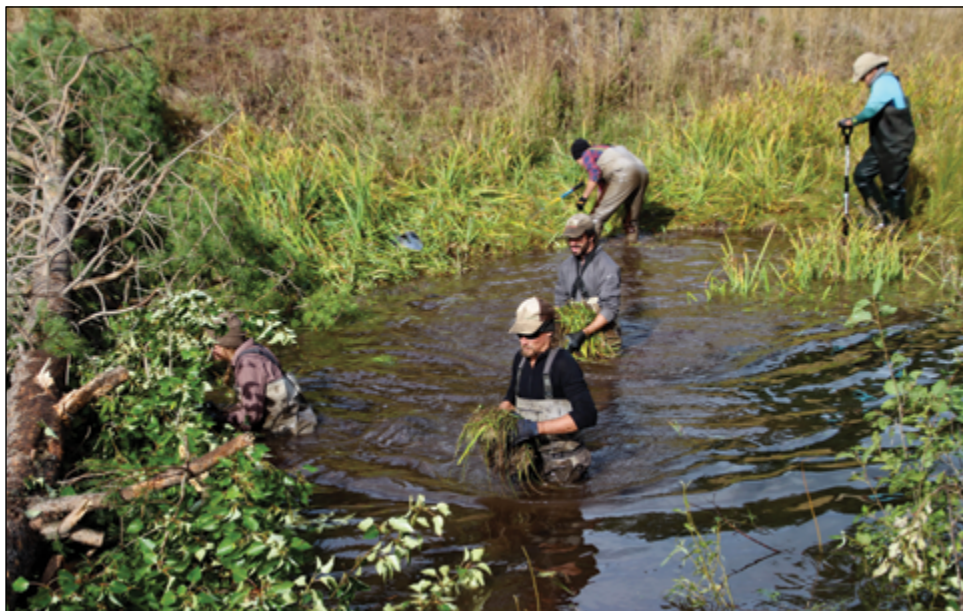
Kevin Swift and his crew designed and installed BDAs on upper Yellow Creek. Photo: Brock Dolman, OAEC.
