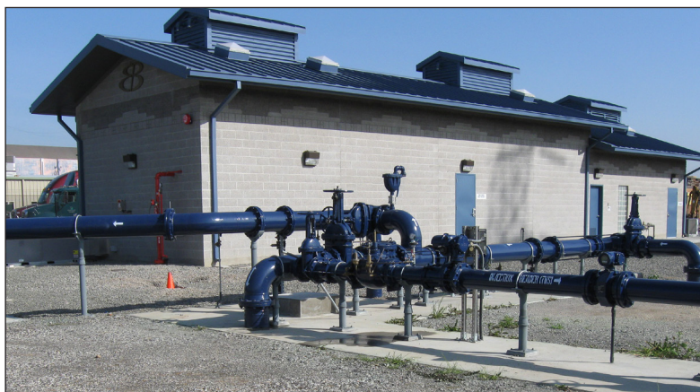
EBMUD'S Bayside Facility. Photo courtesy EBMUD.
