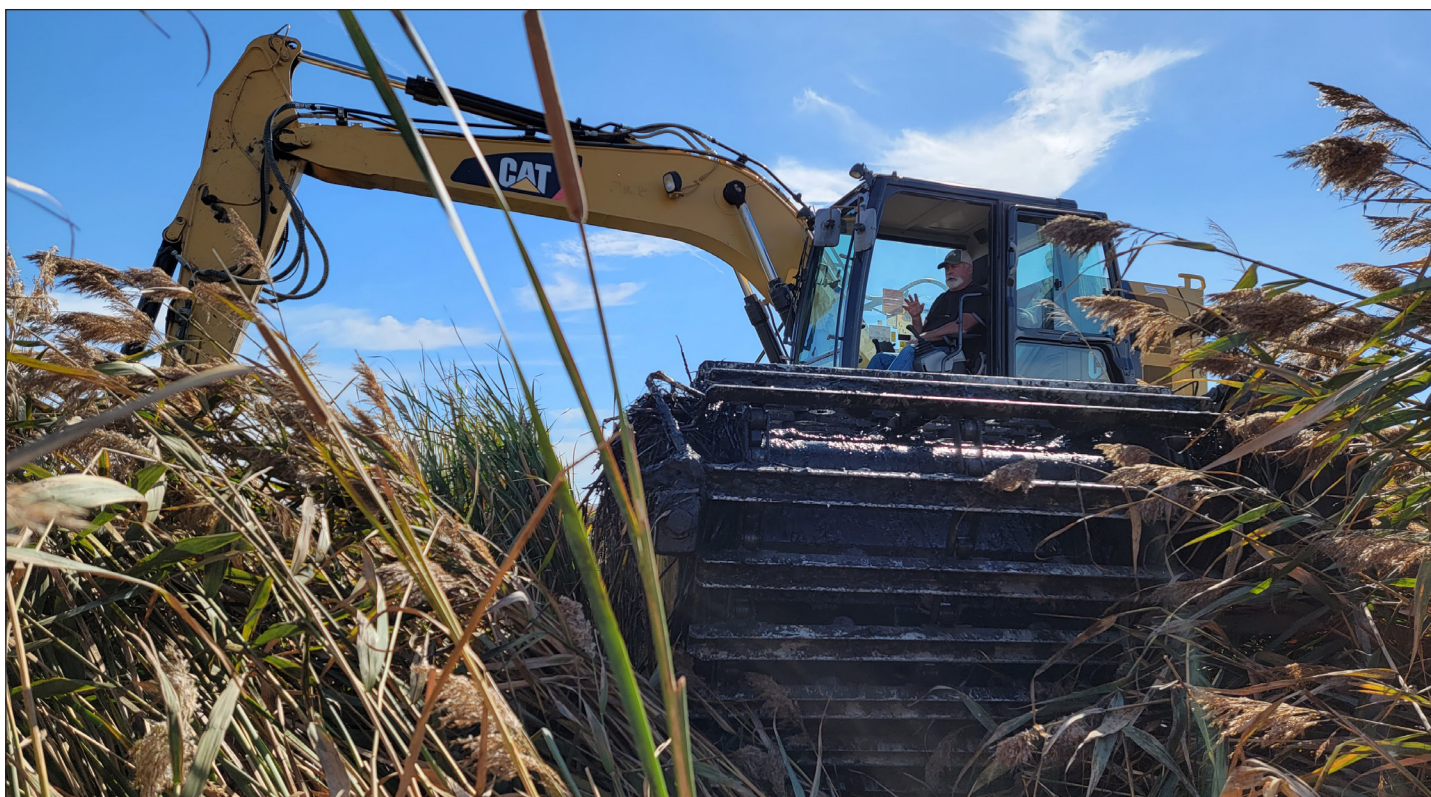
Amphibious excavator, with a lighter footprint on soggy ground, works Hill Slough breach. Photo: Sarah Estrella.
