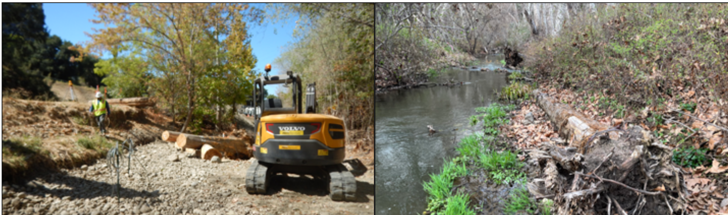
LEFT: Placing spawning gravels on top of creek bottom to improve fish habitat, Los Gatos Creek, 2019. Photo: Valley Water. RIGHT: Woody materials attached to bank by cables, Feb. 2022. Photo: Baykeeper.
