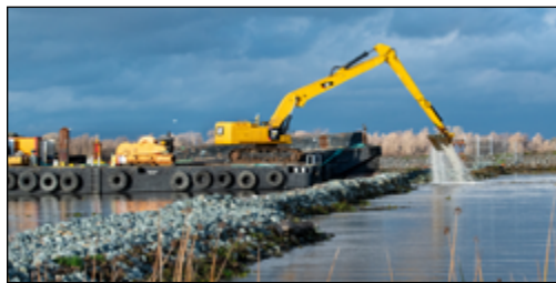
Crews make a notch in the drought barrier in January 2022 to allow fish and vessels to pass through. Photo: DWR
