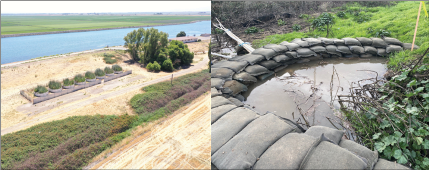
LEFT: Experimental floating wetland cylinders offer promise for fish habitat on the island. RIGHT: Levee boils can cause massive structural damage if not caught quickly. Images courtesy of MWD.
