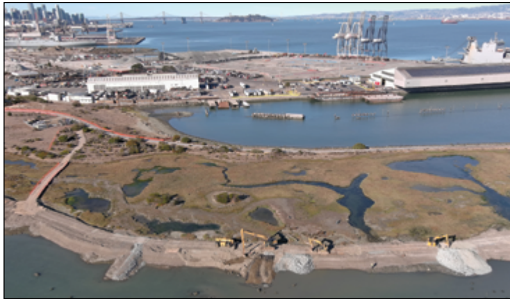
Construction of groins and headlands at Heron's Head in November 2022. Photo: Port of SF
